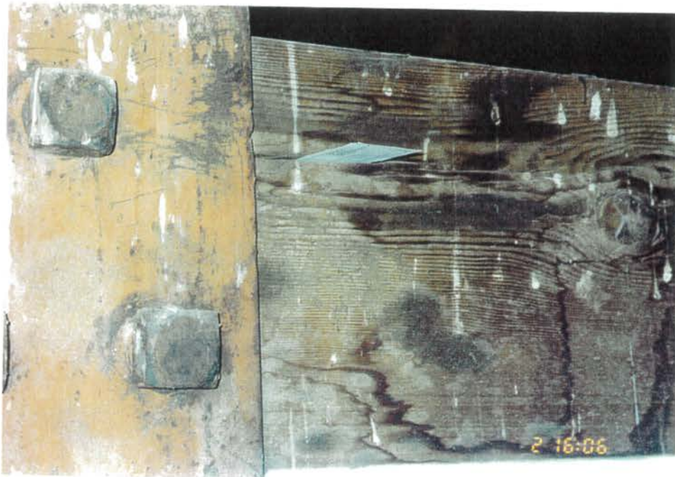
TRUSS E - BOTTOM CHORD SPLIT AT WEST HEEL
