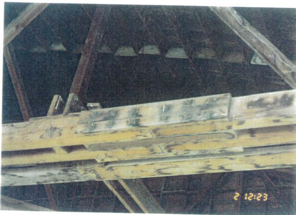
TRUSS B - SPLIT SIDE PLATE AT SPLICE 6
