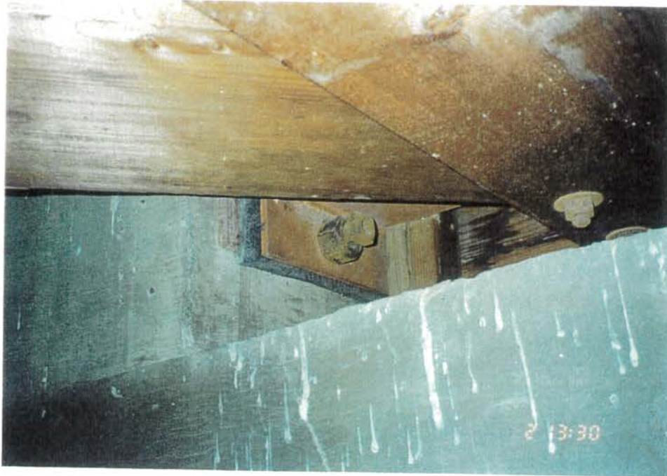
TRUSS F - LOOSE WIND TRUSS ANCHOR BOLT (TYPICAL)
