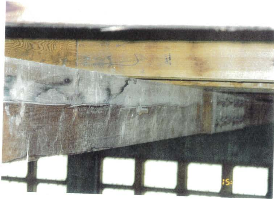
TRUSS D - SPLIT BOTTOM CHORD
