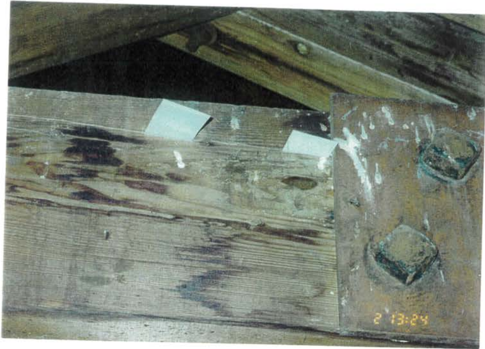
TRUSS B - BOTTOM CHORD SPLIT AT EAST HEEL BOTH SIDES
