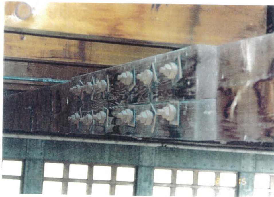
TRUSS C - SPLIT SIDE PLATE AT SPLICE 2
