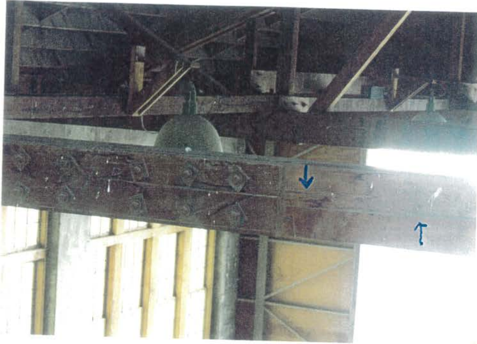
TRUSS D - SPLIT SIDE PLATE AT SPLICE 6 (NOTE: SPLIT BOTTOM CHORD)
