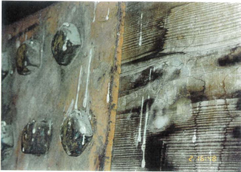
TRUSS F - SMALL BOTTOM CHORD SPLITS AT EAST HEEL
