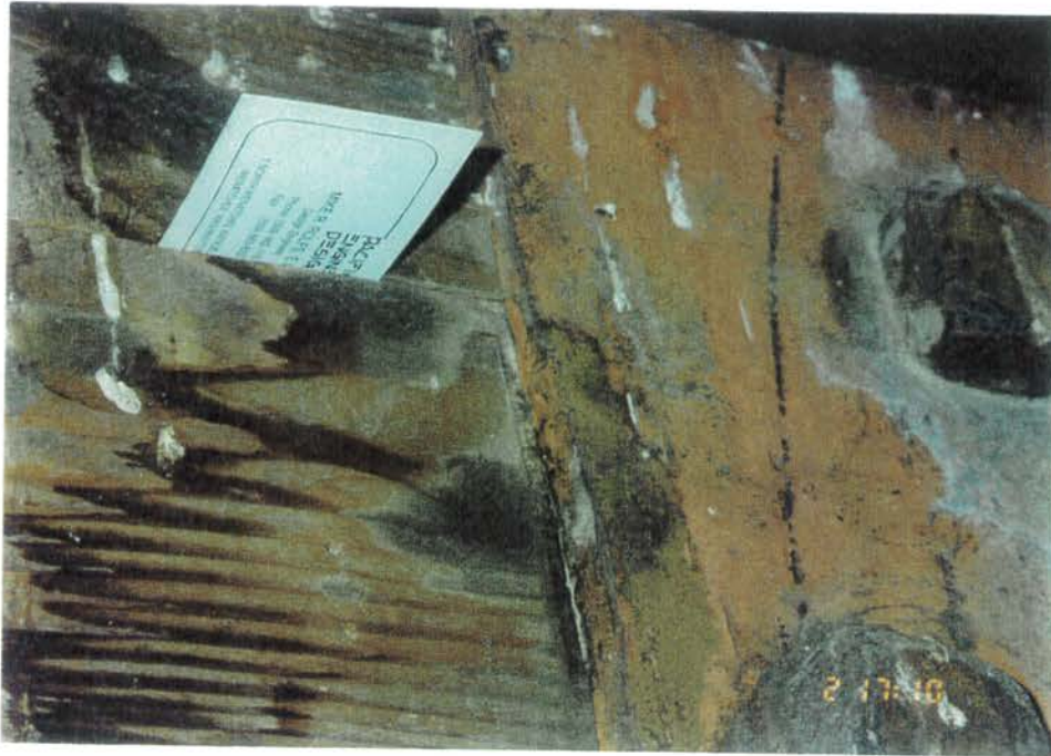
TRUSS F - BOTTOM CHORD SPLIT AT WEST HEEL
