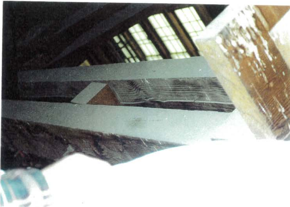
TRUSS B - SPLIT BOTTOM CHORD
