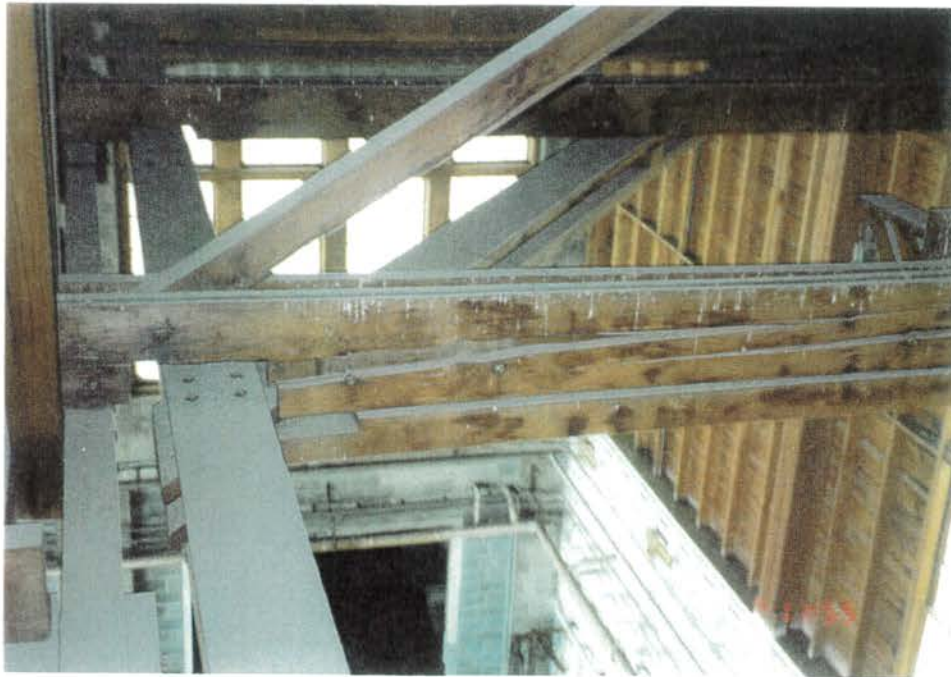
TRUSS B - CRACKED WIND BRACE STRUT
