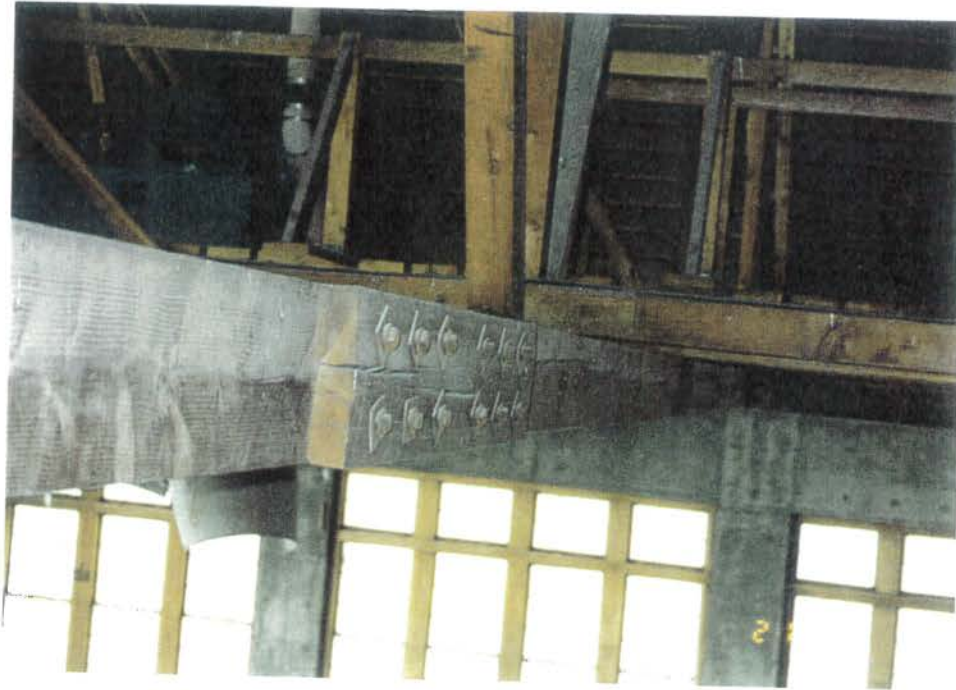
TRUSS E - SPLIT SIDE PLATE AT SPLICE 3 (NOTE: BOTTOM CHORD SPLIT BEYOND)
