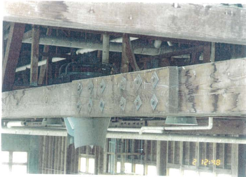
TRUSS C - SPLIT SIDE PLATE AT SPLICE 6
