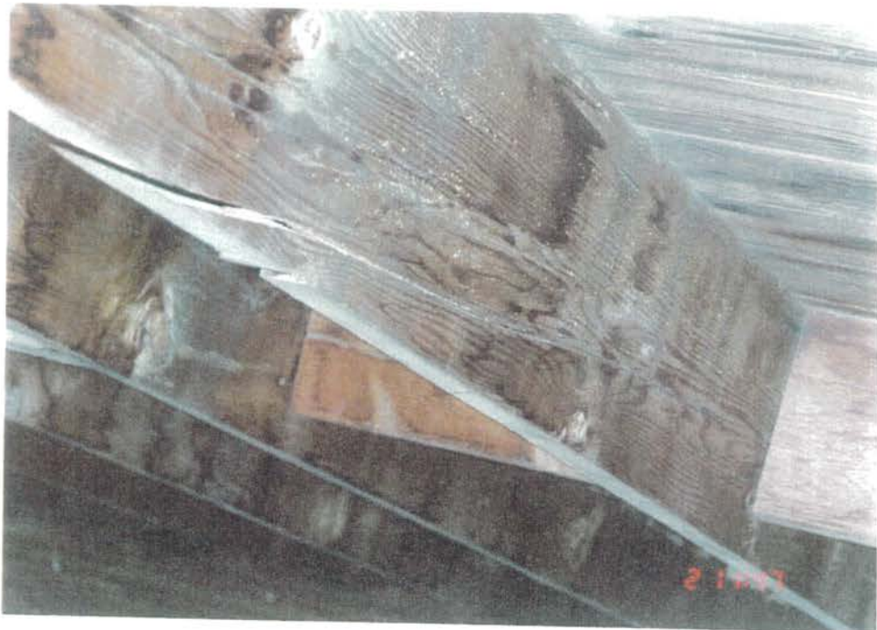
CRACKED JOIST (TYPICAL 5 LOCATIONS)
