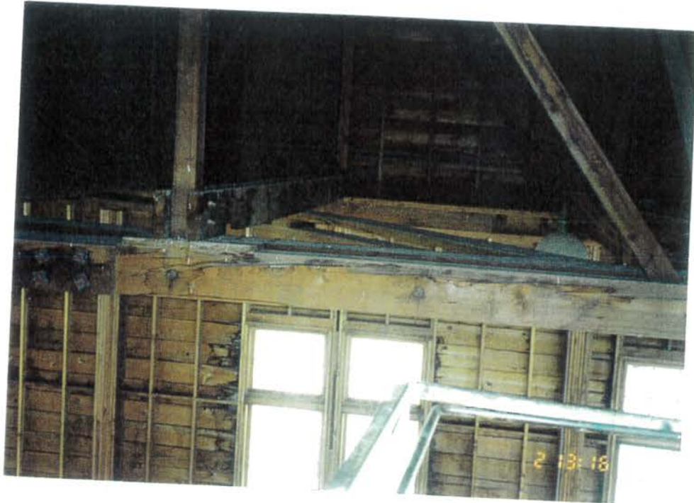
TRUSS B - BOTTOM CHORD SPLIT
