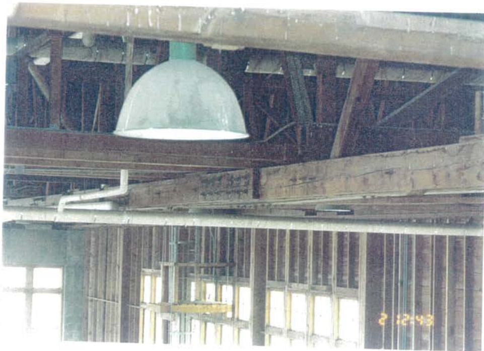
TRUSS B - SPLIT SIDE PLATE AND BOTTOM CHORD SPLIT
