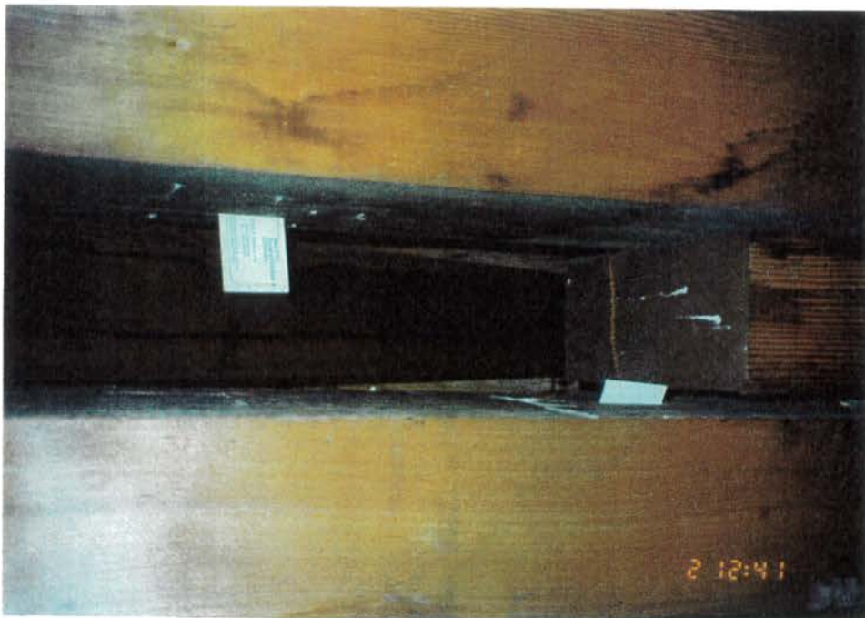
TRUSS C - BOTTOM CHORD SPLITS AT WEST HEEL
