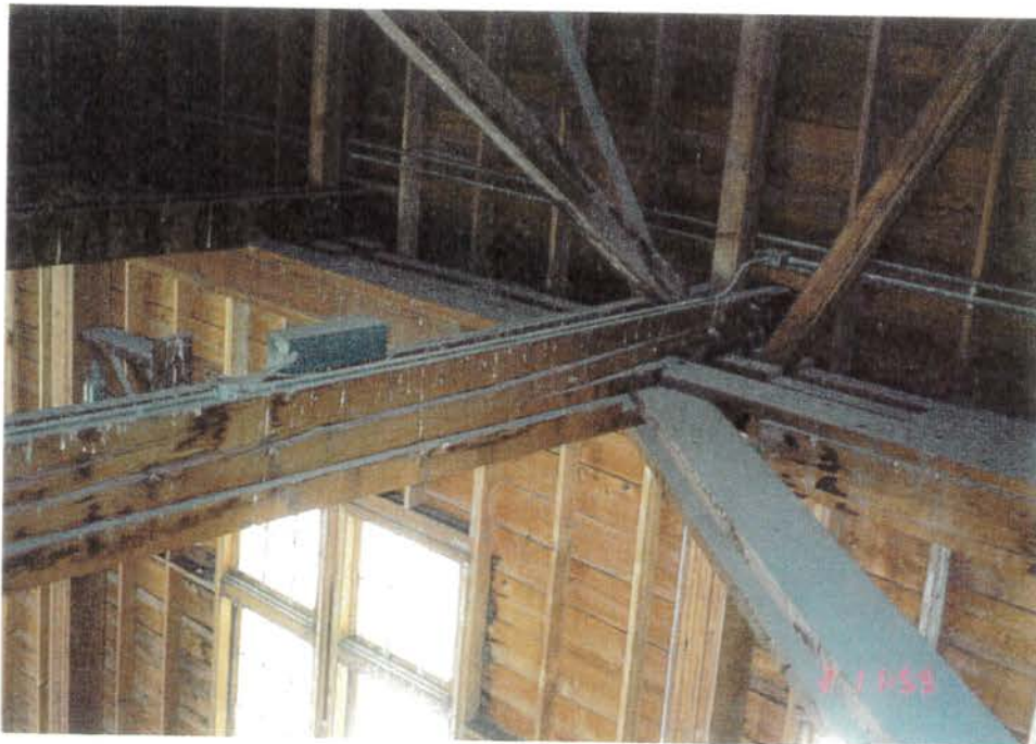
TRUSS A - CRACKED WIND BRACE STRUT
