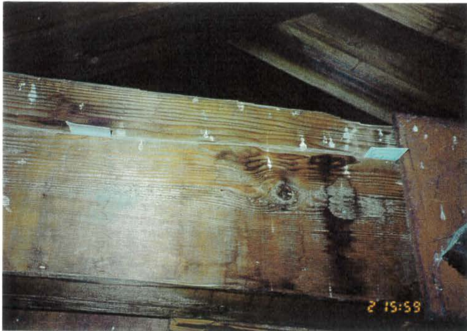
TRUSS D - BOTTOM CHORD SPLIT AT WEST HEEL
