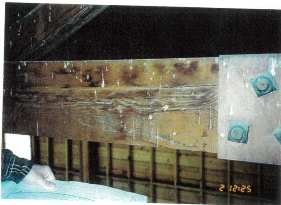
TRUSS B - BOTTOM CHORD SPLIT AT WEST HEEL
