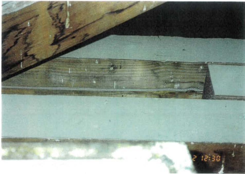
TRUSS B - SPLIT BOTTOM CHORD
