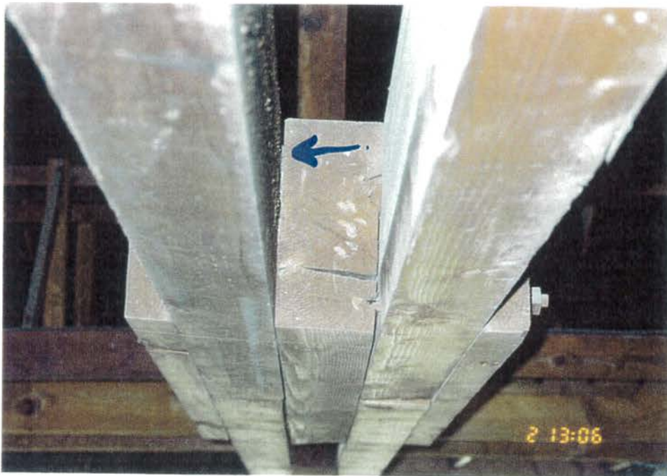
TRUSS C - SPLIT SIDE PLATE AT SPLICE 3 (NOTE: SPLIT RING CONNECTOR IN GAP)
