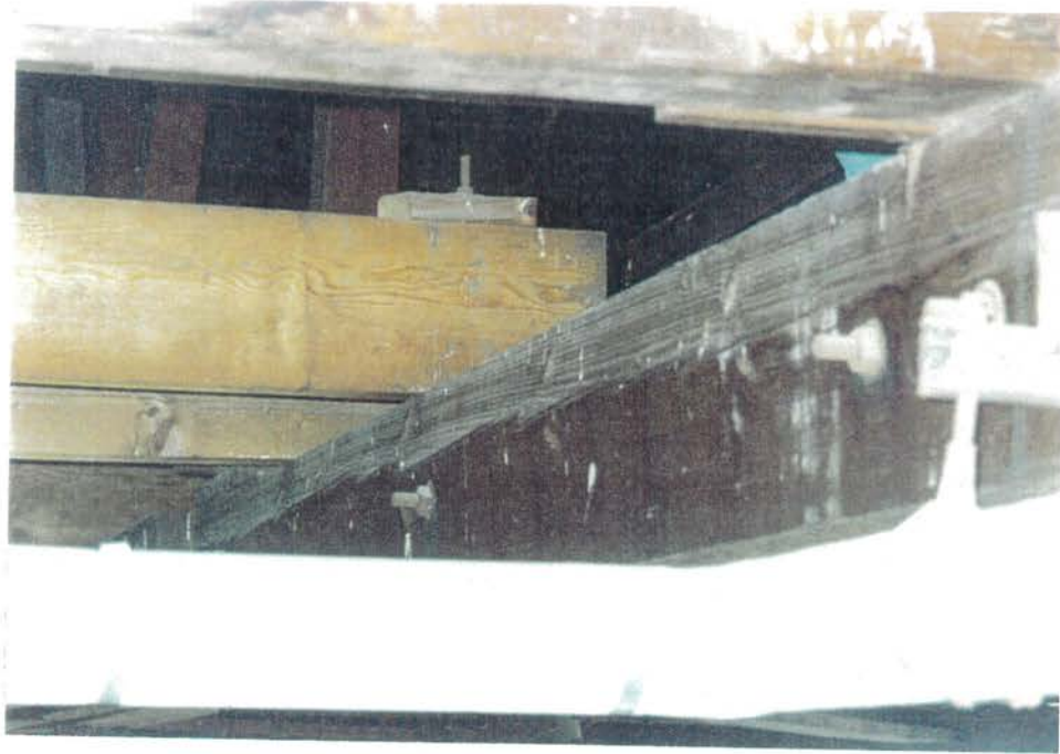
TRUSS F - BOTTOM CHORD SPLIT
