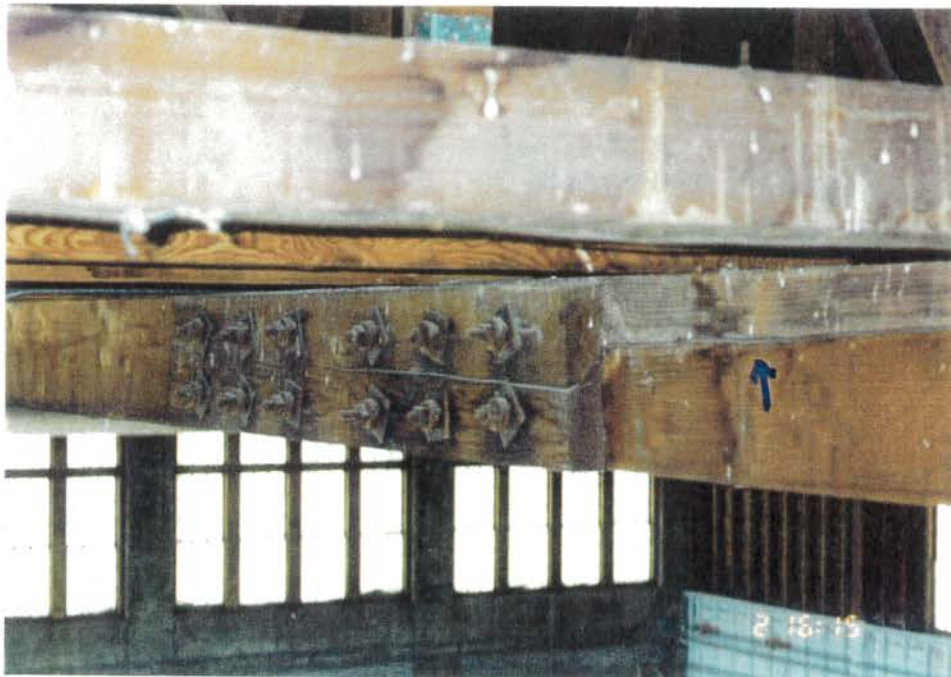
TRUSS E - SPLIT SIDE PLATE AT SPLICE 5 (NOTE: BOTTOM CHORD SPLIT)
