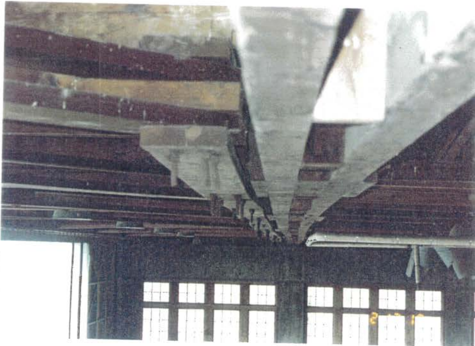
BOTTOM CHORD BOWED
