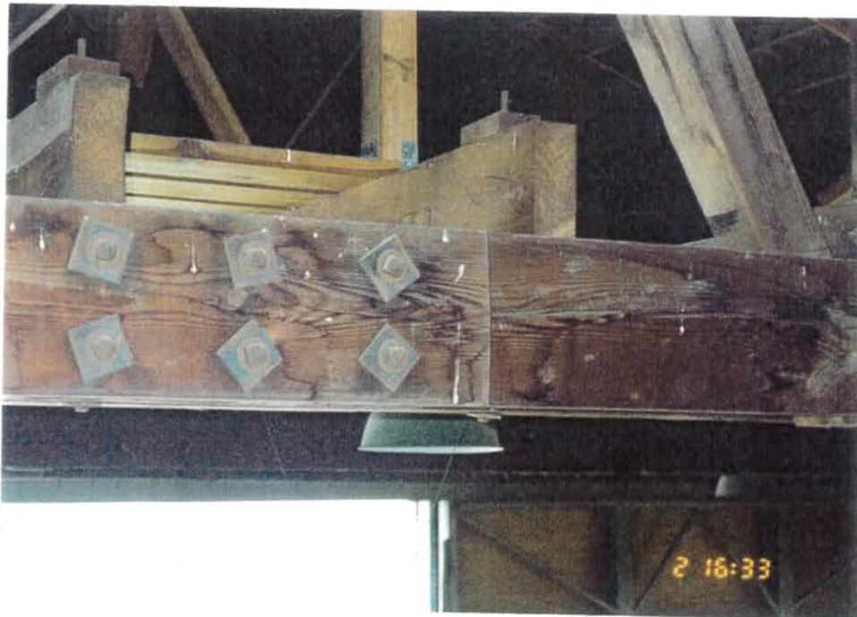
TRUSS E - BOTTOM CHORD SPLIT (NOTE: SMALL CRACKS IN SIDE PLATE)
